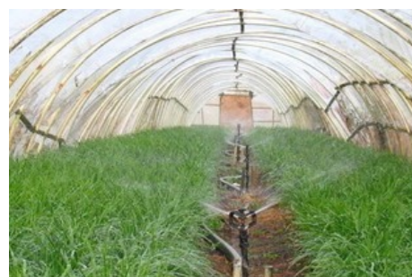
Agricultural greenhouse water supply system
